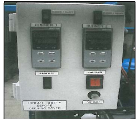
Remote Control from Dive Control Room
